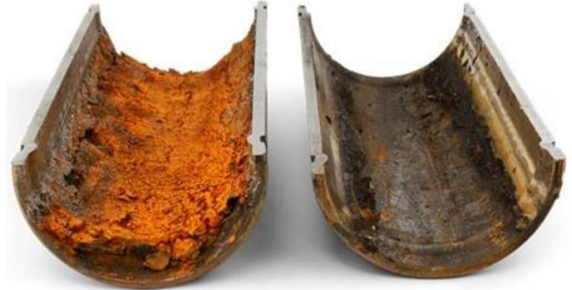
Corrosion on an oil/gas pipeline: a safety related issue.
